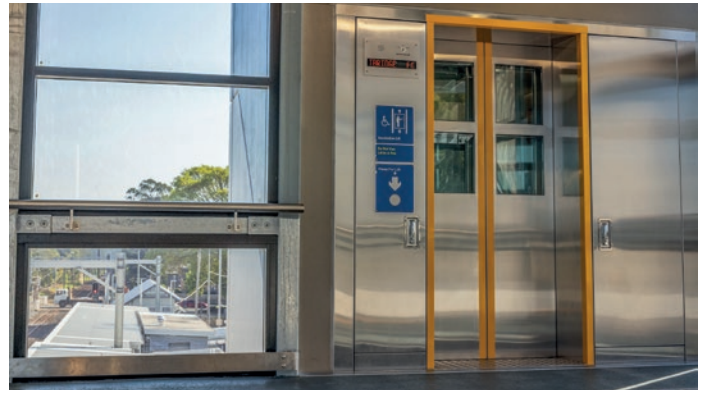
Lift access to platform
