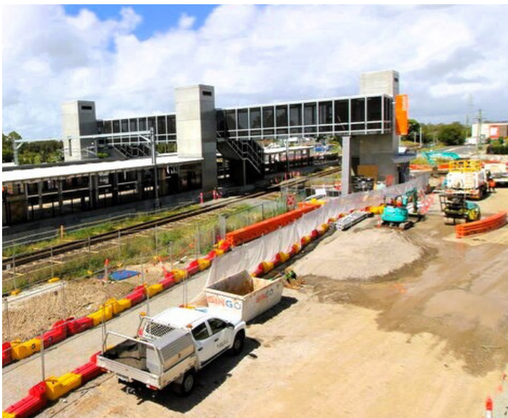
Above: New Lindum station platforms and footbridge, with North Road carpark expansion works.
